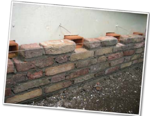
The system installed in a new to build house. Ceramic elements are visible.
